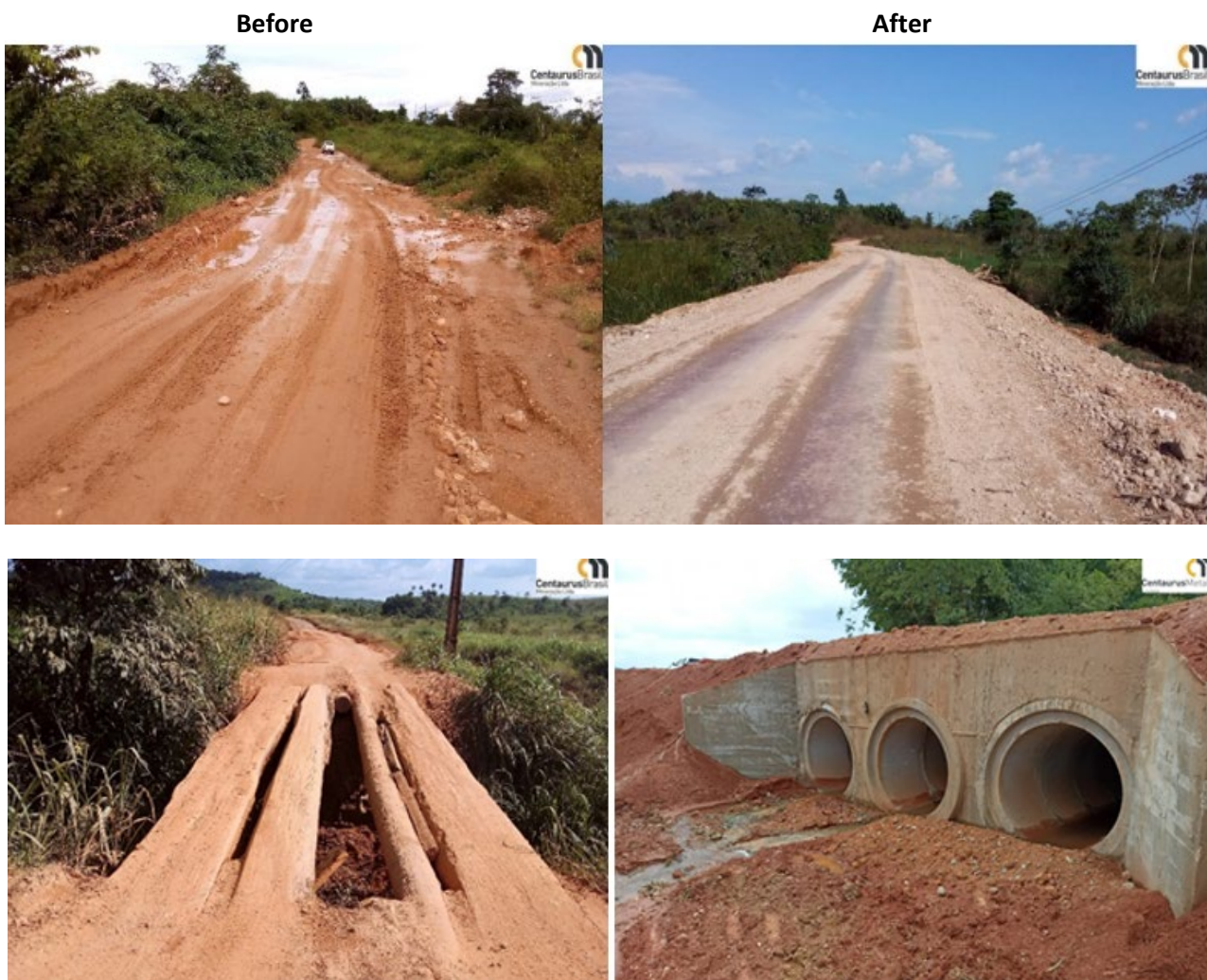
Figure 7 – Road Upgrade Work completed as a result of the Public Private Partnership with the Sao Felix do Xingu Municipality
