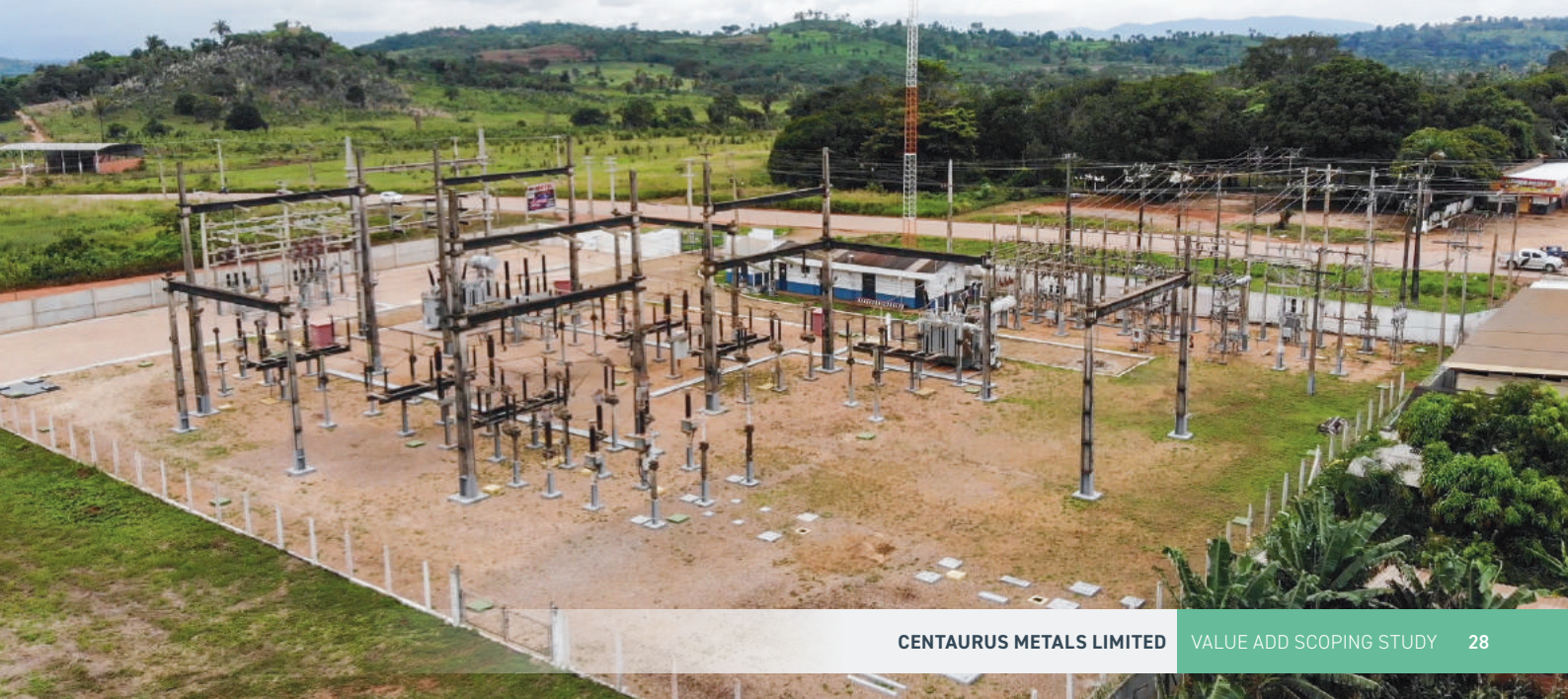
Figure 19 - 138kV National Grid connection at Tucumã
