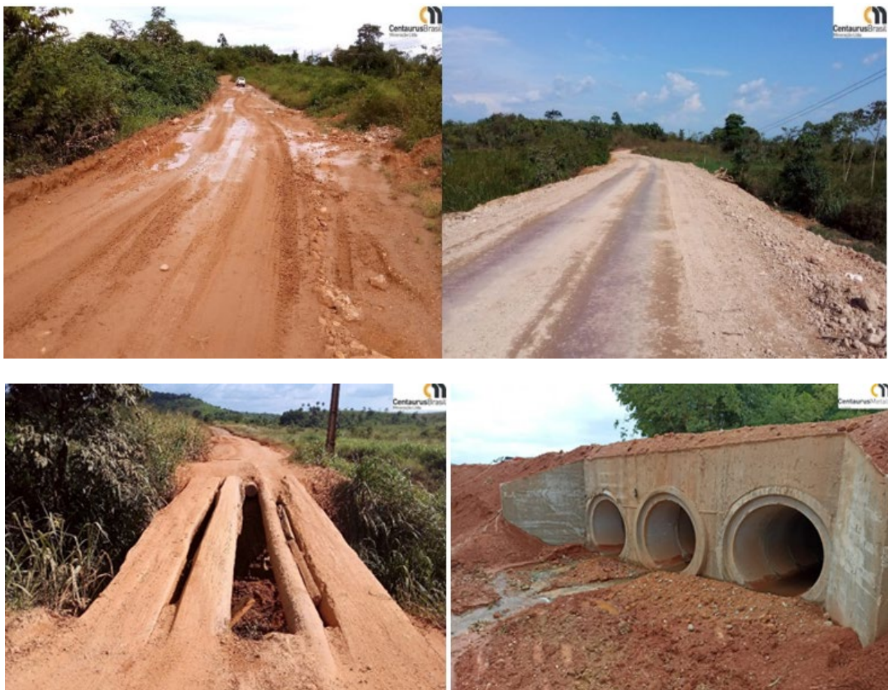
Figure 6 – Road Upgrade Work completed as a result of the Public Private Partnership with the Sao Felix do Xingu Municipality
